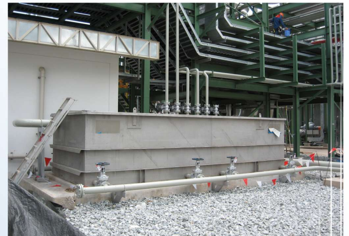
Thai Shinryo – 60 m3/h Oil Separator
