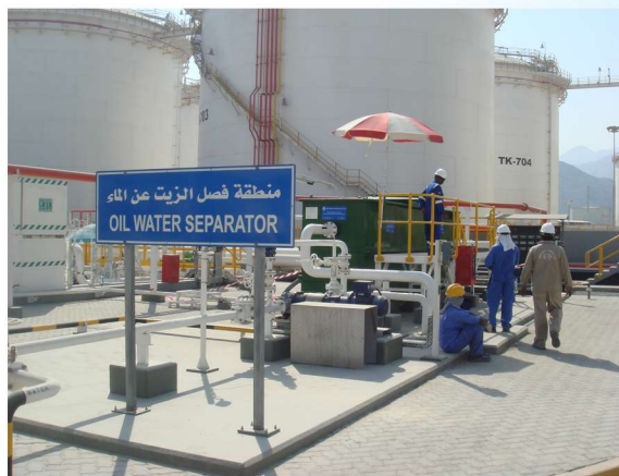
Oil Terminal, UAE - 1,200 m3/d
