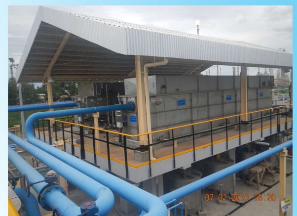
Oil Refinery, Indonesia - 4,320 m3/d
