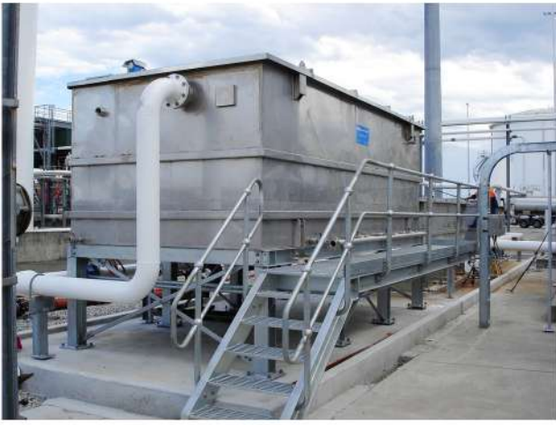
Fuel Terminal, Sydney - 2,800m 3 /d
