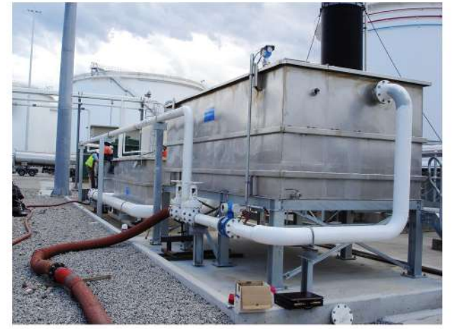
Fuel Terminal, Sydney - 2,800m 3 /d
