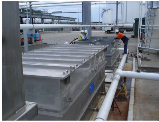
Fuel Terminal, Sydney - 2,800m 3 /d
