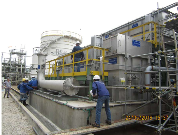
PTTGC I4 Olefin WWTP – 50 m3/h DAF & Oil Separator
