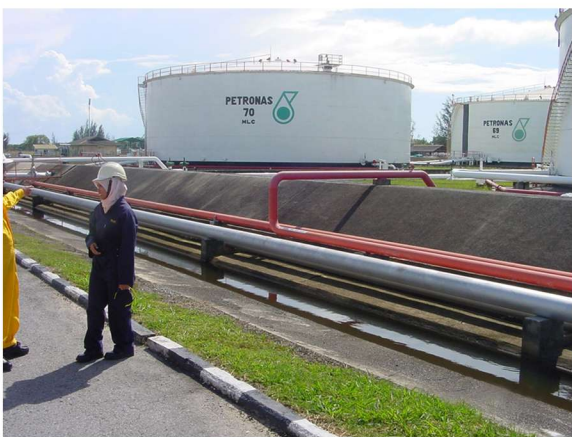
Fuel Terminal, Malaysia - 36,000 m3/d
