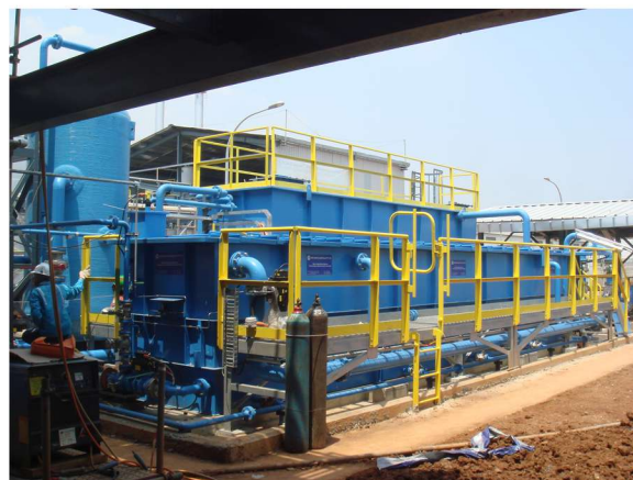
Shell Monas Lube Oil Blending Plant Jakarta, Indonesia 60 m3/hr
