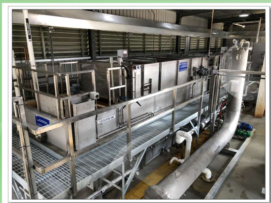
Inghams Plant, Ingleburn 20 m 3 /h
