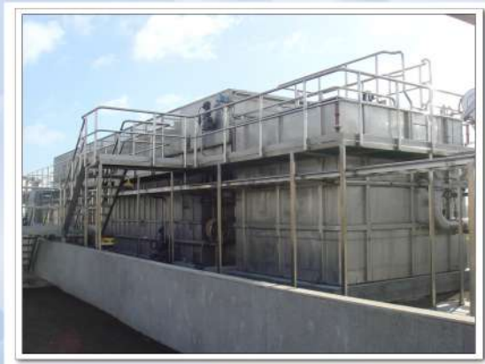
Fonterra NZ – 250 m3/h DAF Plant
